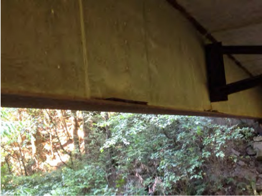
delaminating on bottom flange
