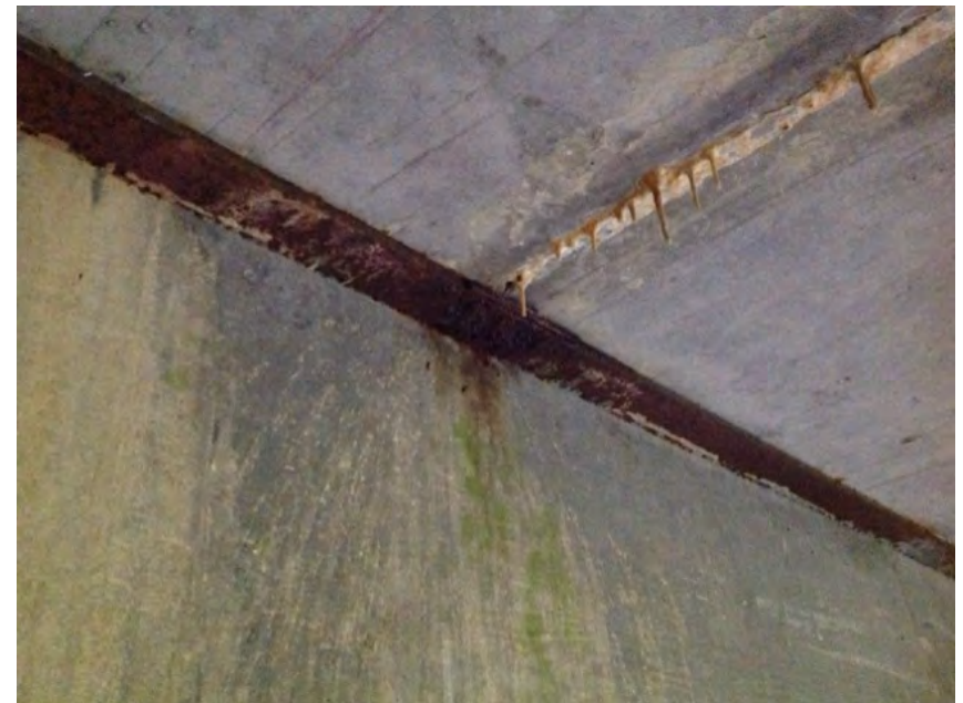
water getting through at deck joint
