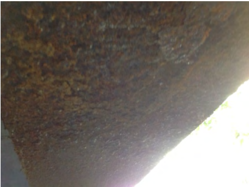
more delaminating on bottom flange
