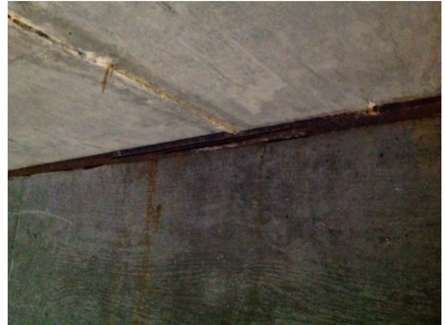
some delaminating of the top flange at deck joint
